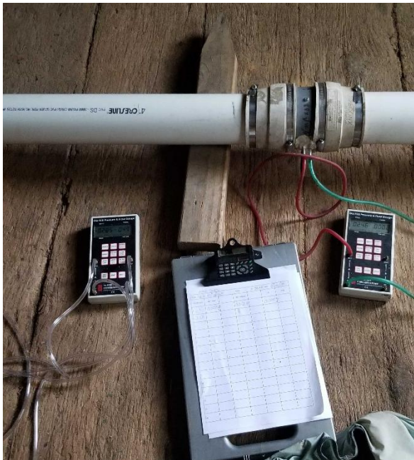
Figure (15): Five-inch flow grid used to make 4" PVC airflow measurements
